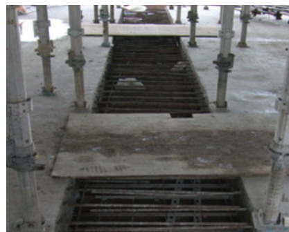
Pour Strips restrict site access, cause a trip hazard and delay progress on site
