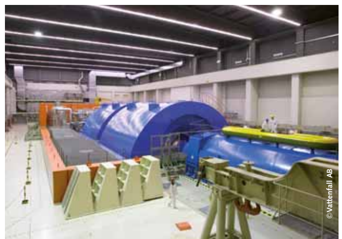
Turbine block in a nuclear power plant
